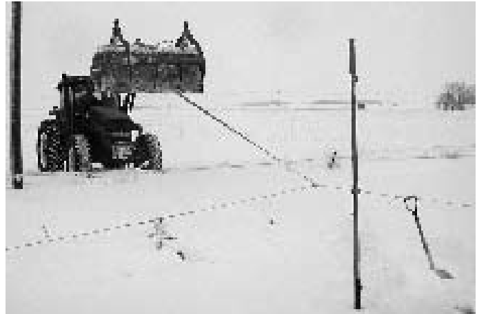
Not only did local farmers do a great job plowing roads and providing access to poles, they also were invaluable in lifting power lines. Lines were literally frozen to the ground, and then buried by several feet of snow. Here, Tim Krcil uses a little horsepower to rip the wire out of the snowbank, to be re-strung on the pole.
