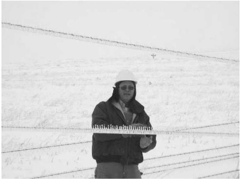
Rod Payer demonstrates how thick the ice accumulations were on this downed power line. This line was south of Wagner, not far from Jerald Ehrisman's farm.
